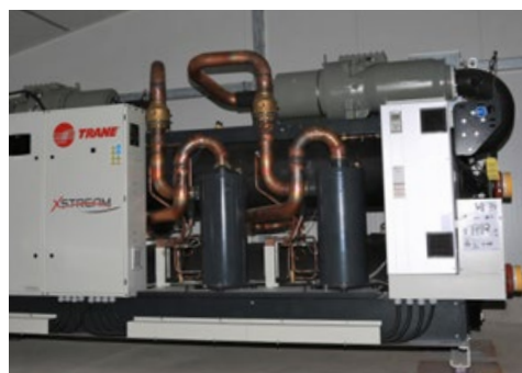
The new heat pump at SKF Steyr.
